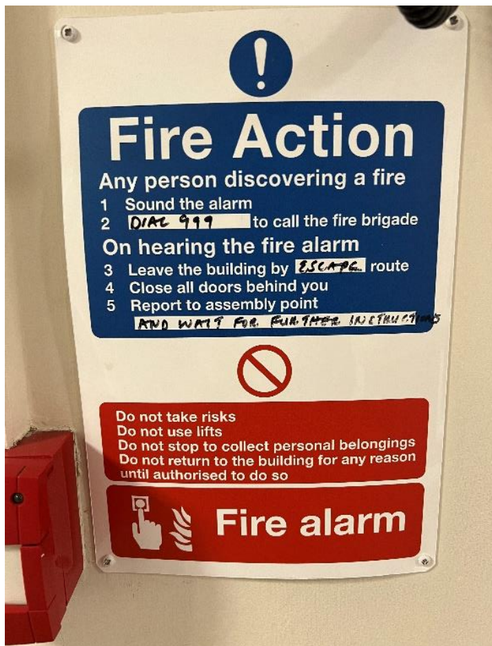
Figure 3. Appropriate fire safety information was displayed consistently throughout the premises.
